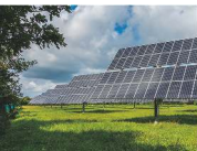
Solar Pumping System
