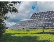
Solar Pumping System
