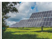
Solar Pumping System
