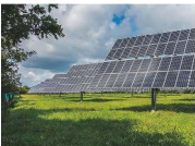
Solar Pumping System
