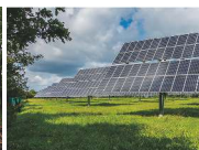
Solar Pumping System
