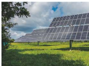
Solar Pumping System
