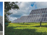
Solar Pumping System
